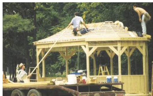
Workers assemble the gazebo behind Pattison Lodge in 1992. The Lodge and gazebo are home to more than 100 weddings every year.
